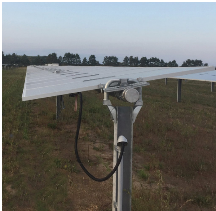
Badger State will use a panel design similar to the image above
